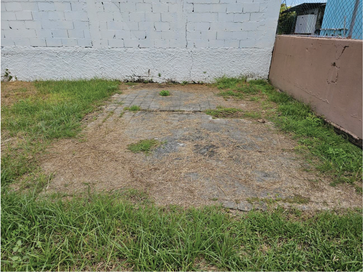
Photograph 7 – Concrete floor with tiles. According to a neighbour, there was a septic system at this area.
