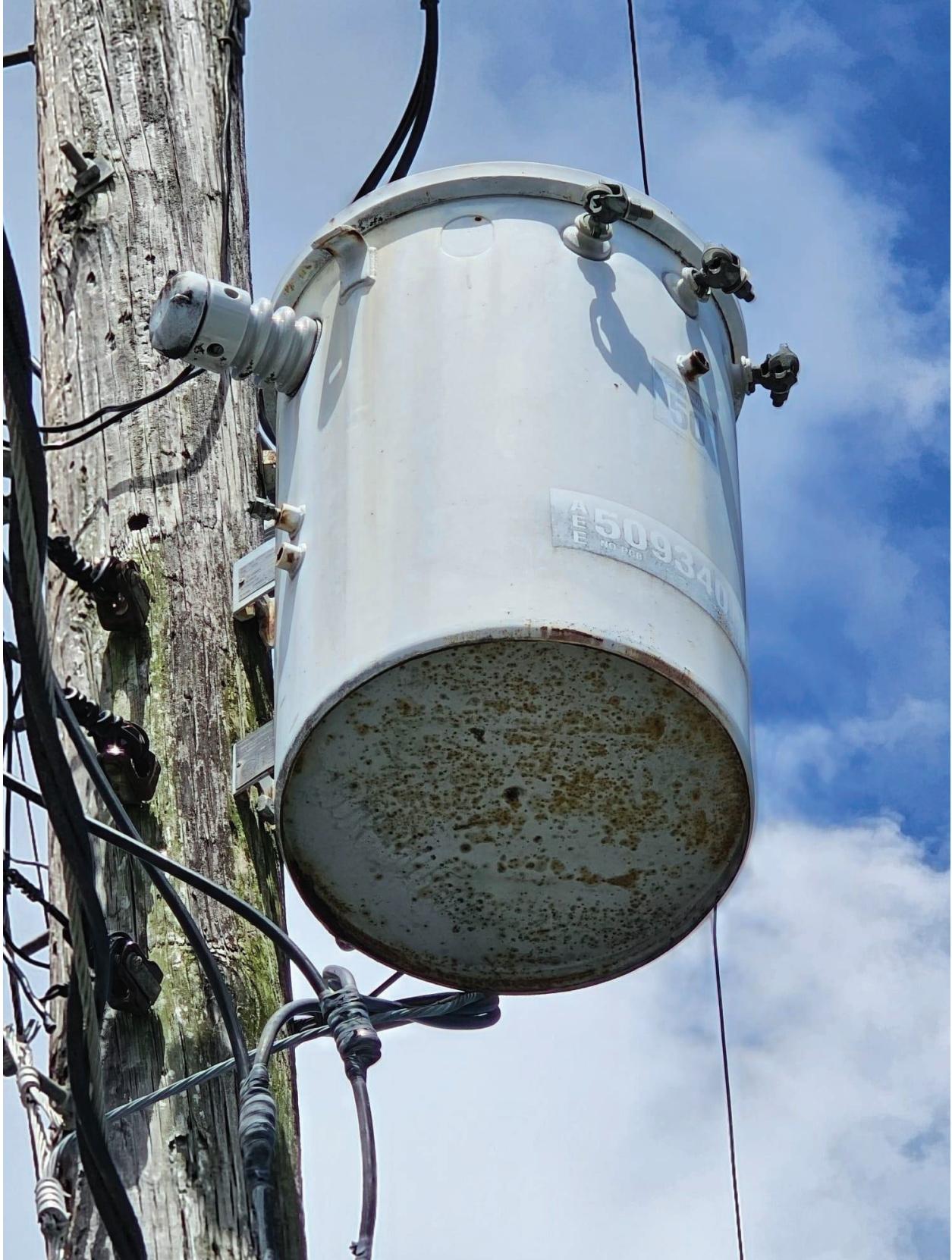
Photograph 6 – Electric transformer with faded No PCB sign.
