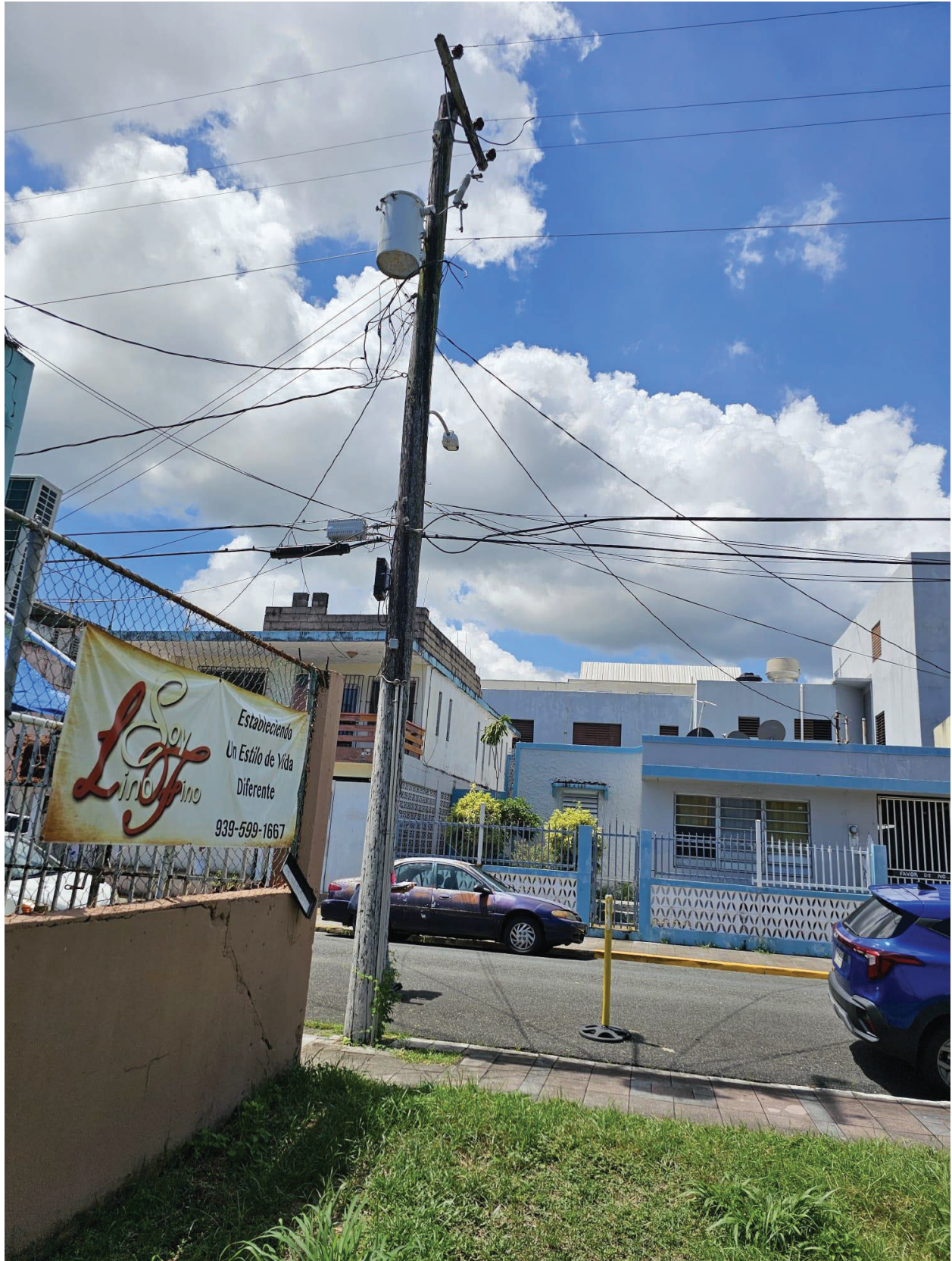
Photograph 5 – Electric transformer at pole located at the southwestern corner.
